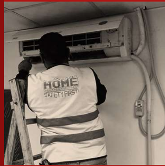
Air Conditioning Units
